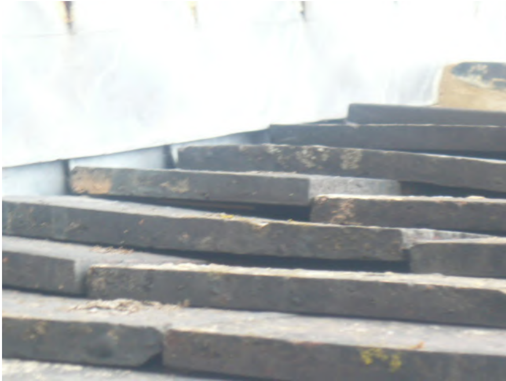
Photograph 4: Tiles adjacent to the central chimney that are not sitting correctly viewed from the South West.
